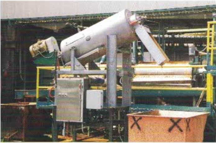
FF-12 FILTERING WASTEWATER AFTER DRUM SCREENS
