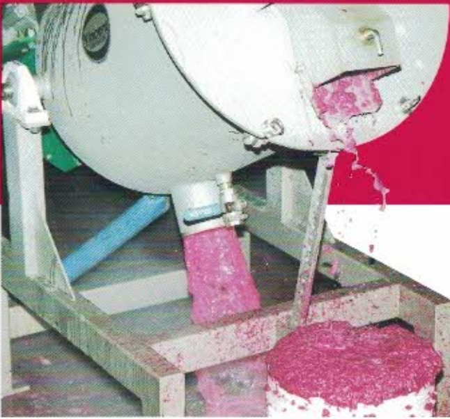
SLUDGE DISCHARGE INTO 5-GALLON PAIL
