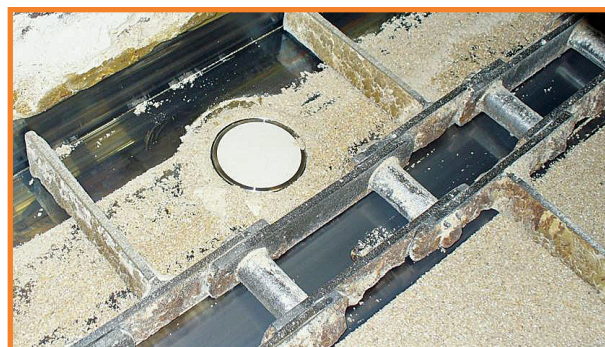
Measuring moisture of animal feed in conveyor
